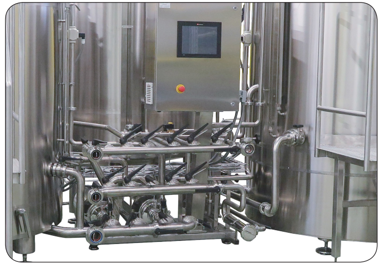
Pipeline with pumps and valves
